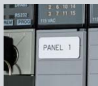
Control panel labels
